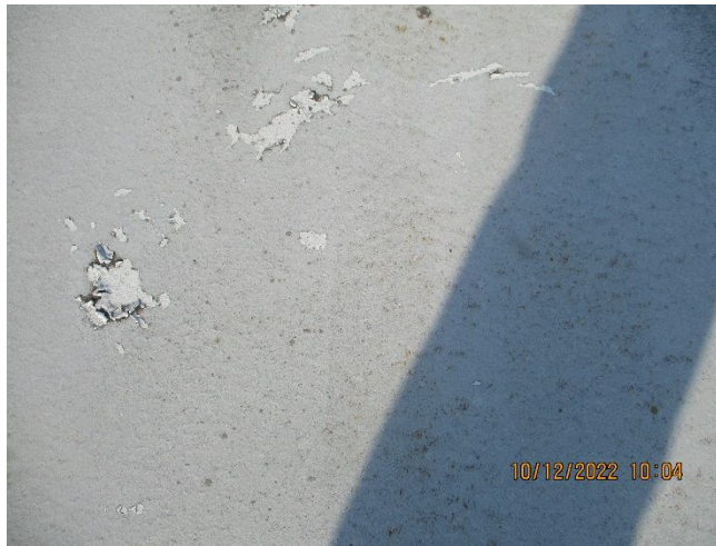
PHOTO 2 small areas of delamination
