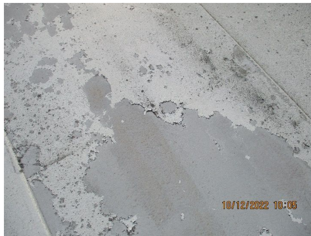
PHOTO 3 Delamination of Topcoat
