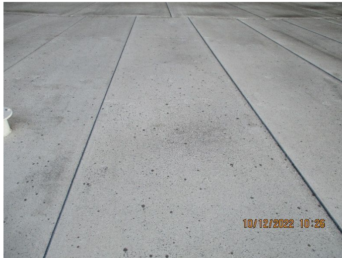
PHOTO 8 View of Random spots of Delaminations of Topcoat
