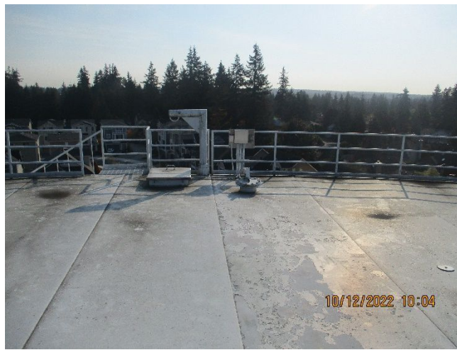
PHOTO 1 Example of Topcoat delamination
