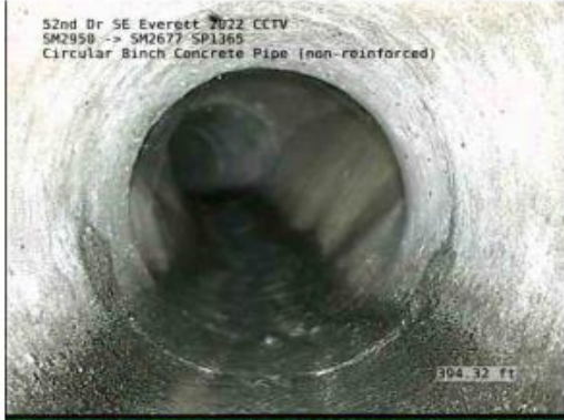
SP1365-FC-394.324890136719 .jpg, 00:23:04, 394.32ft Fracture Circumferential from 12 o'clock to 12 o'clock
